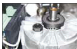
Electric motor and gears in oil lubrication
